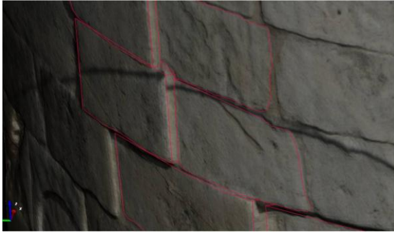
Figure 4: Particular of the dislocation of ashlars of the main apse of San Pietro church, Coppito, L'Aquila, Italy.
